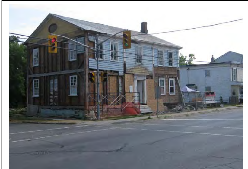
Rehabilitation and restoration work on the Ham House (353 Main Street) is able to identify historic construction methods, as well as articulating the importance of quality materials and craftsmanship
