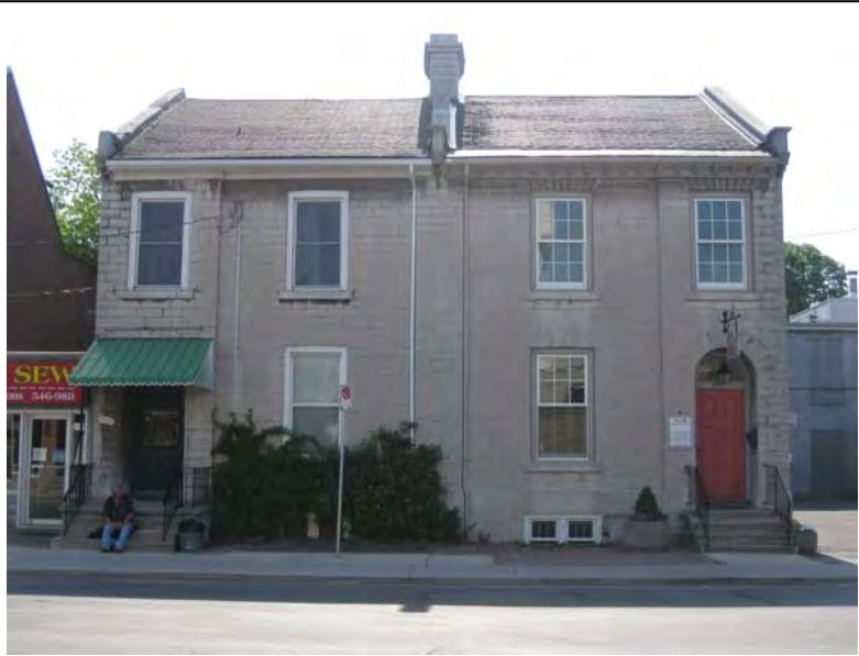
Heritage-quality windows are integral to the cultural heritage value of many heritage resources. On the right, heritage-quality windows have been conserved. On the left, windows have been replaced, with a significant impact on the physical or design values of the heritage resource.
