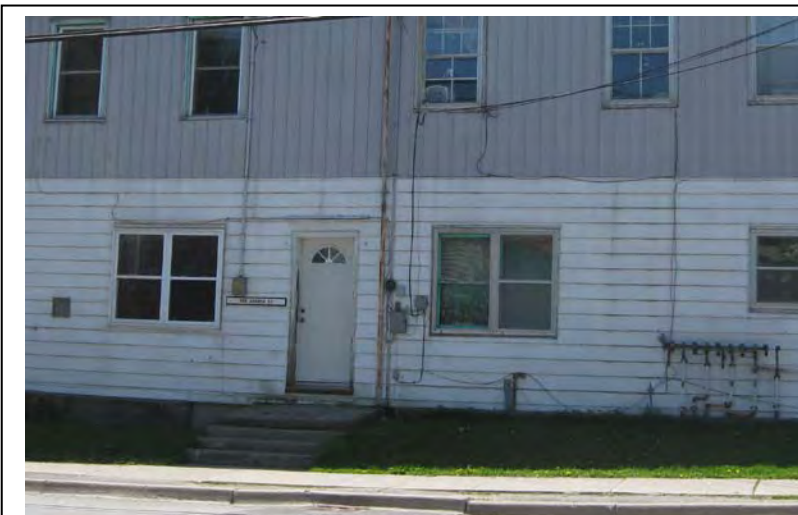
The placement of utility meters on the Church Street façade of 195 Church Street negatively detracts from its cultural heritage value. The utility meters clutter building, interrupting the symmetry of the façade. The rear of the building would be a more appropriate location for utility meters.
